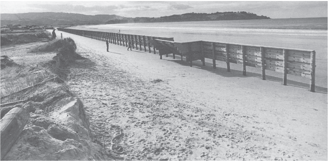
(Above): During storms in 1975 and 1976, sand and maram grass were removed from behind the “protective” wall, and the sea started cutting into beach-front sections. Note the stranded stairway, part way along the wall, which used to lead onto the grass. Photo courtesy of Cliff Grant.
